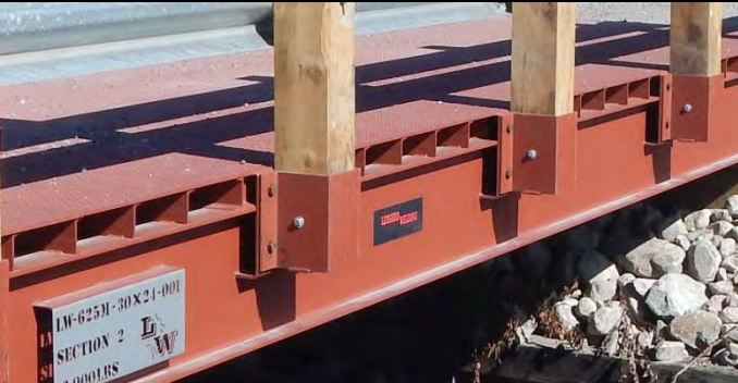
Photo 5: Close-up of post pocket anchors used to provide TL-1 barrier system on NEW 9.2m span x 7.1m wide modular bridge. Bridge ID Plate also visible.
