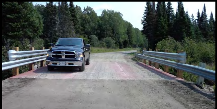
Photo 8: Looking Southerly at full deck width of new 9.2m span x 7.1m wide Lessard Modular bridge.
