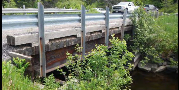
Photo 2: Downstream face of existing 9.2m span stringer bridge with laminated timber deck covered with excessive granular materials (Barrier system in place does not meet Code or 2016 MTO Exceptions document).
