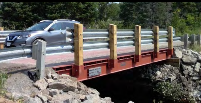
Photo 7: Downstream face of NEW 9.2m span x 7.1m wide modular bridge - installed in a single day over newly installed bridge bearings.
