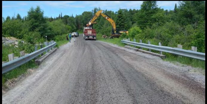
Photo 4: View looking northerly of existing 9.2m span stringer bridge. New modular bridge being offloaded in the background.
