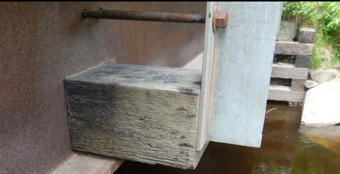
Photo 3: Close-up of barrier base showing 8 x 8 block held in place by 25mm threaded rod. Threaded Rod also 'acted' as an intermediate diaphragm/spacer.
